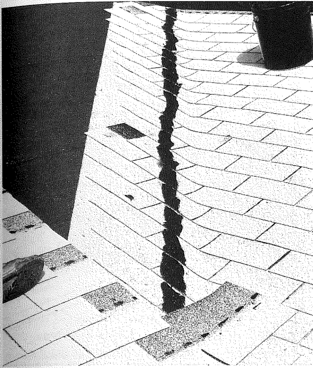
Figure 4-33 Shingle at least 12 inches onto the adjoining roof plane. Note the roofing cement.
